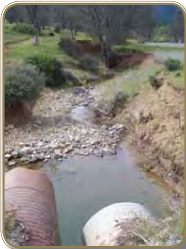
Downstream view before culvert upgrade shows severe erosion. If old, undersized culverts failed, upstream stretch would suffer similar erosion.
